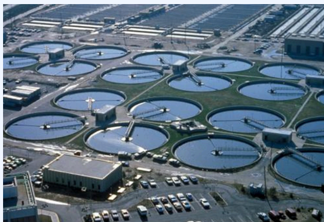
Figure 17.6d: Wastewater treatment facilities, such as this one, remove contaminants from wastewater before the water is released back into the natural environment. (credit: work by eutrophication&hypoxia, CC BY 2.0)
